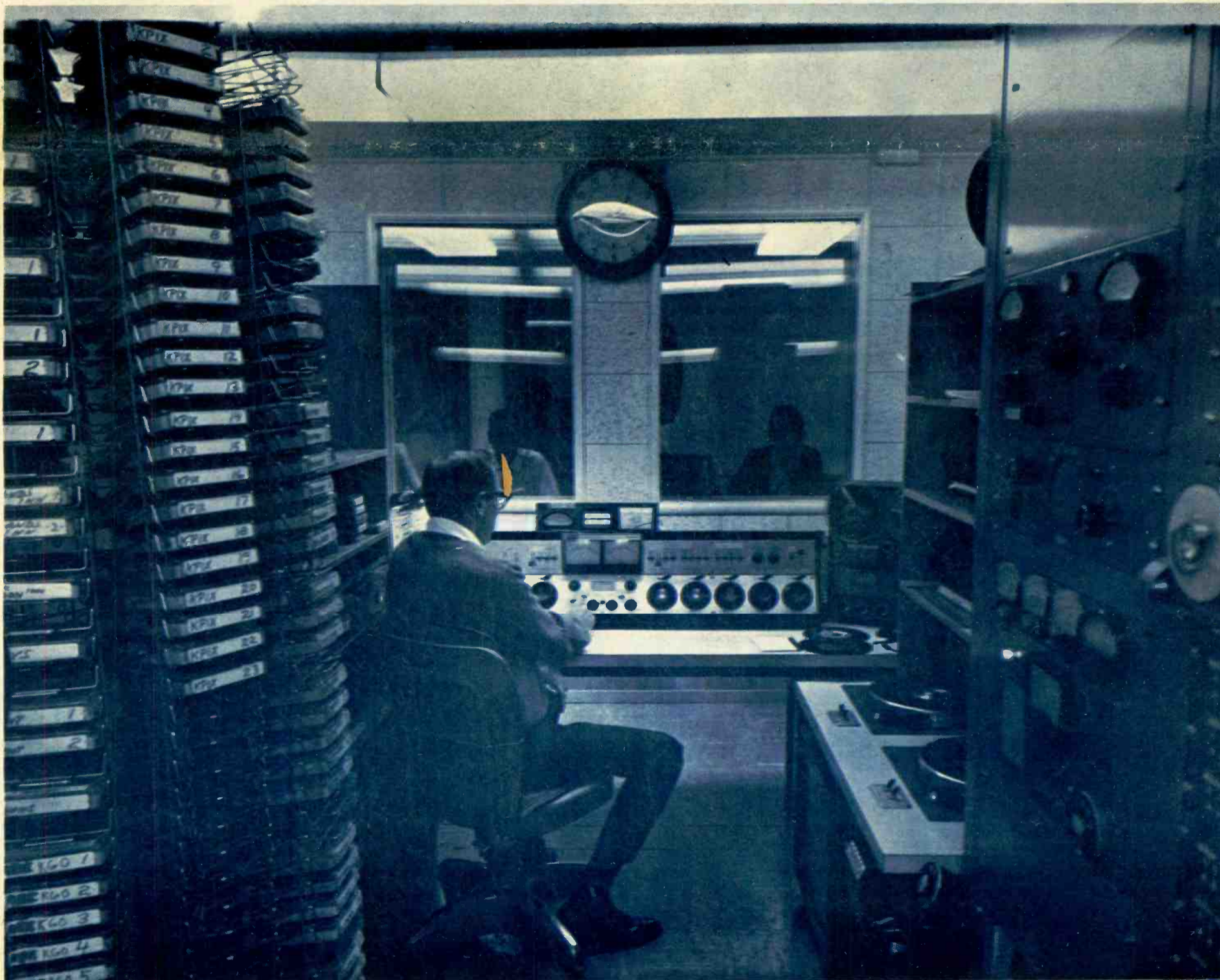
Engineers using this ultra-modern facility at KEWB's new JACK LONDON SQUARE studios look directly into the studios used by KEWB's BOSS MEN, and the KEWB NEWS STAFF. In this photo the engineer sits at the latest transistorized mixing console which "mixes" the announcer's voice and the music. On the right is technical equipment used for the careful monitoring of KEWB's giant transmitter facility. And on the left, are tape cartridges of commercials heard on Channel 91. Take note of that clock in the center — it is synchronized with the National Bureau of Standards in Washington, D.C. Thus, KEWB is always giving you the official right time, as kept by a government agency.
