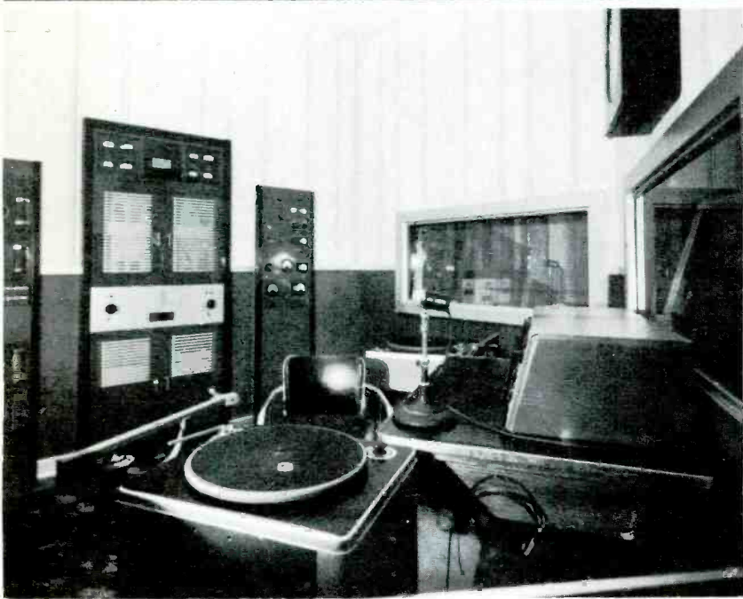
TRANSMITTER AND MASTER CONTROL ROOM. Behind the grills on the wall is KFDA's new transmitter. White panel in center pulls down for access to transmitter control panel. Small "mike" in foreground is "talk-back" to studios.
