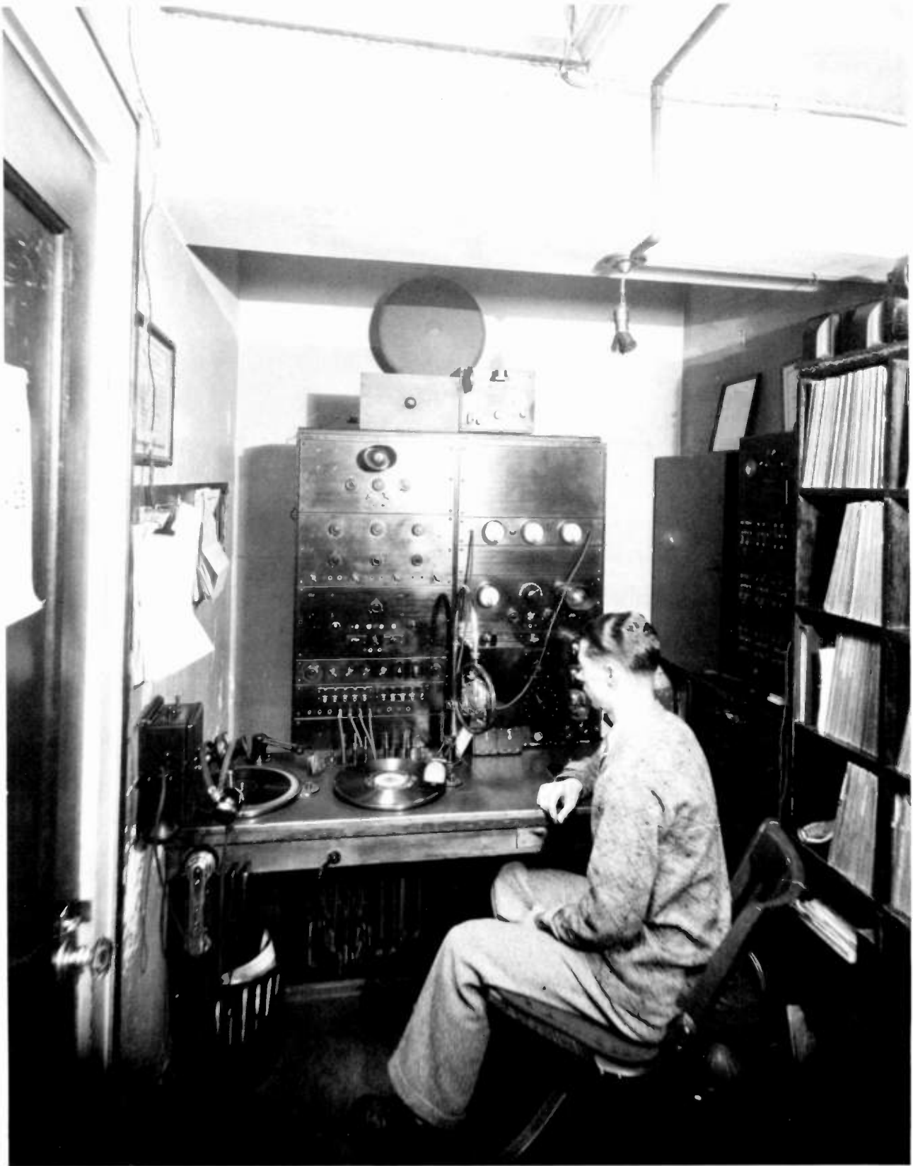
Control room for KVOS , Bellingham, in 1930. The operator on duty is H. Ben Murphy . Note the telephones and switchboard, used to talk with the studio announcer and to place remote broadcasts on the air.
