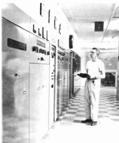
Technician Dave Naff reads the meters on 50 kw transmitter.
