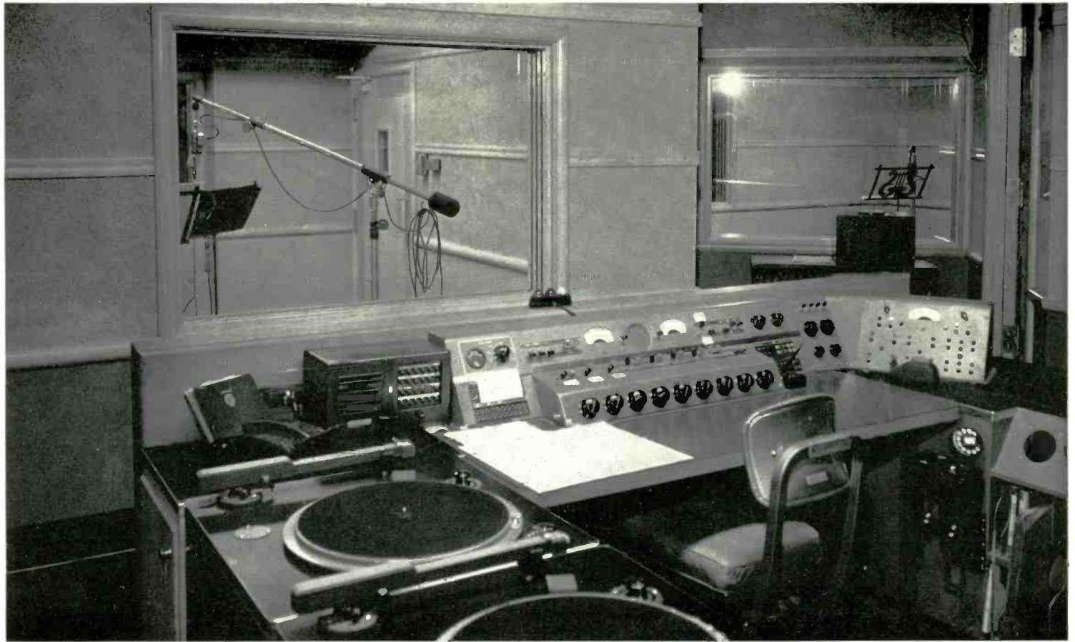
MASTER CONTROL DESK SHOWING SPECIALLY BUILT SWITCHING CONSOLE AND TRANSCRIPTION TURNTABLES
