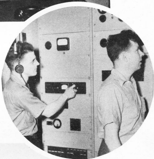
Routine check at the transmitter. Technicians are JACK E. HUMASON (left) and IRVING B. GRANT.
