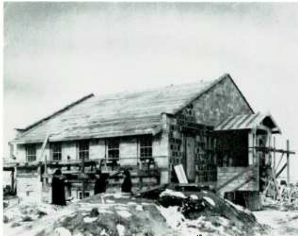
Ground-breaking ceremonies at the site of the new WCCO transmitter in Anoka were held in October of 1924 and this photo of the construction of the building was taken early in 1925.
