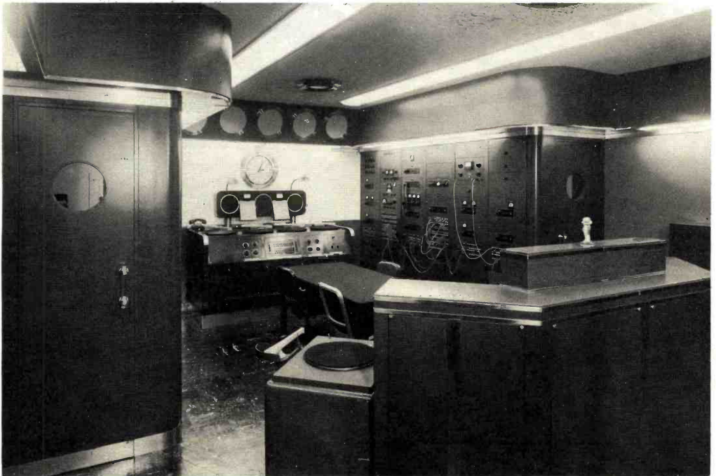
The WJR master control room for AM and FM is the nerve center for all engineering operations of the station.
