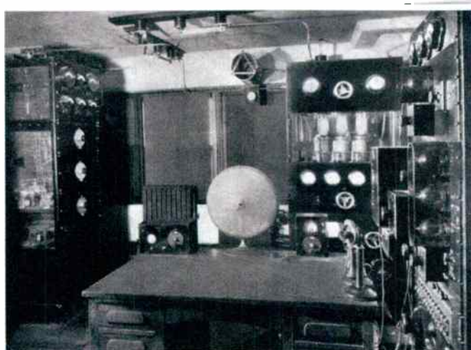
KMA transmitter room, 1927.
