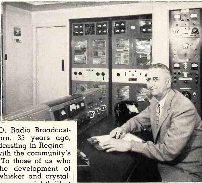
ERNIE STRONG, Chief Engineer, CKCK Radio and CKCK-TV, seated at a control panel in CKCK Radio's Transmitter.
